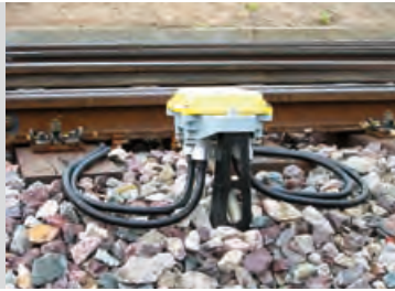
PMAFIX/PMAFLEX in exterior applications (Points heating equipment)
