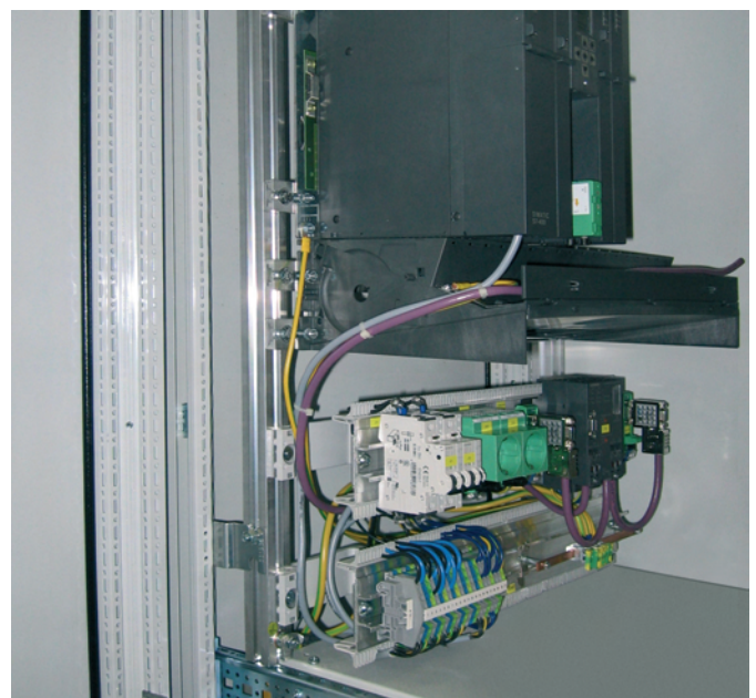
LSC-BRACKET system in the programming cabinet
