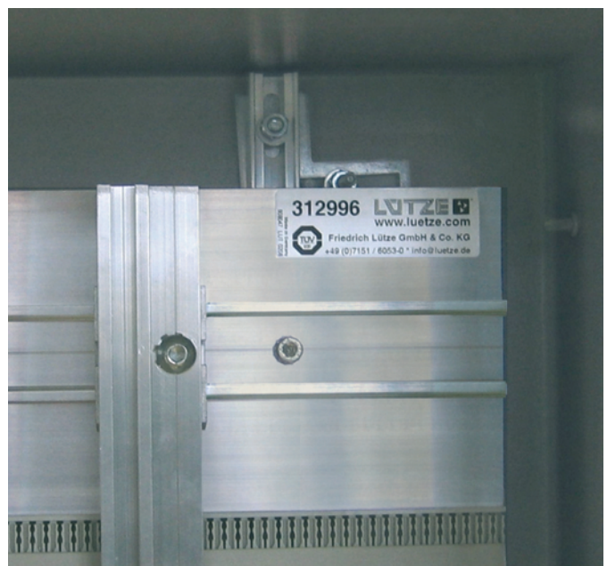
Installation situation in the CM housing
